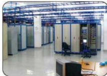
IDC engine room
